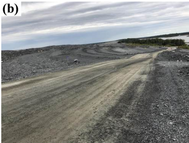
Figure 1. (a) Waste rock pile and (b) mining haul roads made of crushed waste rock at Canadian Malartic mine site, Quebec, Canada
