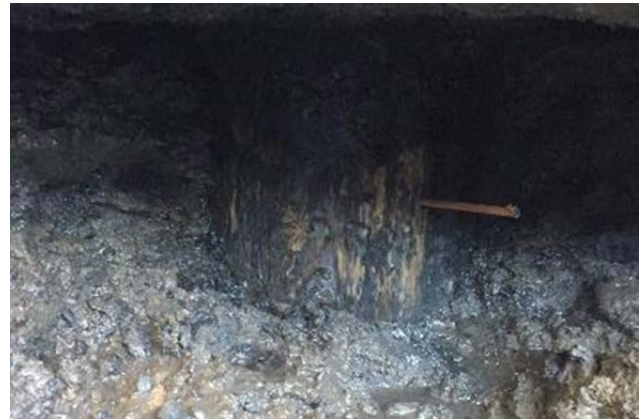
Figure 6. An exposed timber pile.
