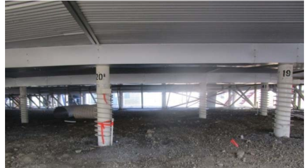
Figure 1. Helix thermopiles under a building in Inuvik, NWT.
