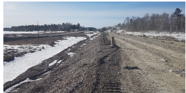
Figure 2. Photograph of the Swamp 305 southbound lane embankment with surcharge in place, facing south from north limits
