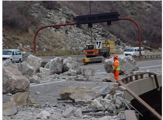
Figure 3. Rockfall on I-70 highway through Glenwood canyon in Colorado, USA. Photo: Colorado Department of Transportation.
