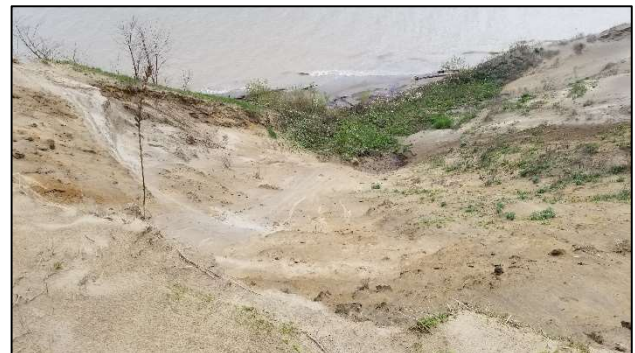
Figure 2. View of the bluff face from which seepage can be seen discharging. Limited vegetation is visible at the toe, along with downed trees.
