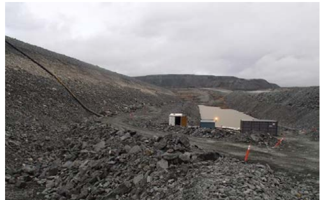
Figure 1: Picture of the downstream pond at the toe of the dike formed by seepage and pumping station
