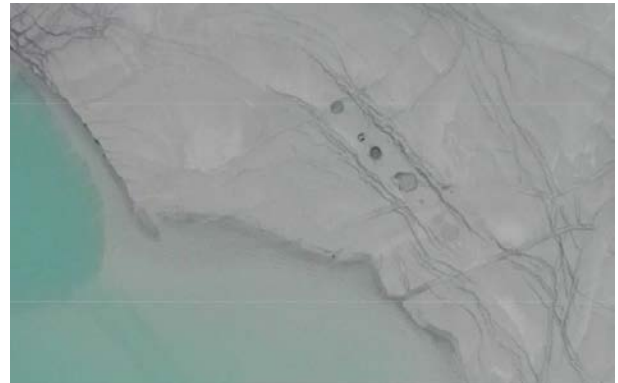
Figure 4: Localized tension cracks and circular depression features in the tailings surface, indicating entry points into the underlying foundation
