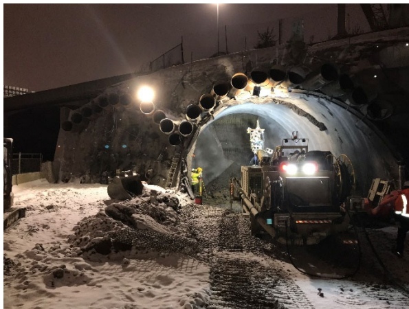
Figure 1. Photo of construction taken from East Portal showing the pipe canopy roofs have been installed for both tunnels.
