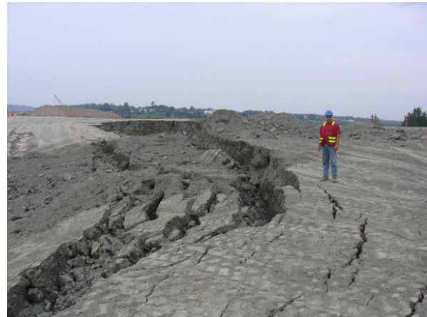
Figure 1. Embankment Failure Condition, July 2006
