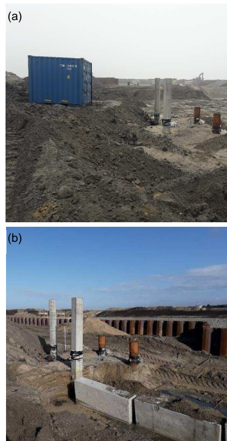
Figure 6. Test site at (a) Day 78 and (b) Day 126 (before placing the 3.0 m fill). The concrete slabs in (b) are anchor plates for the sheet pile wall seen in the background.
