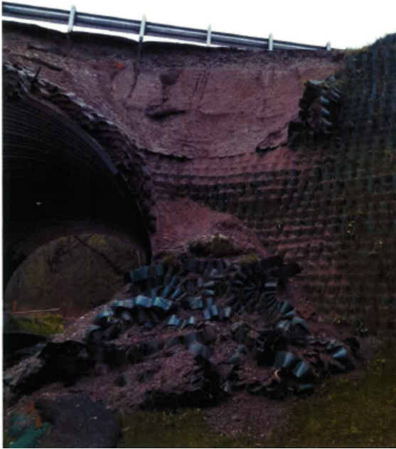
Photo 1. Failure of reinforced soil slope at Culvert A
