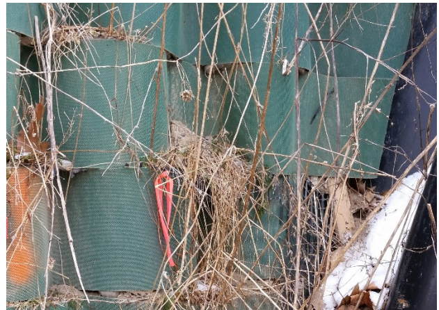
Photo 2. Local soil erosion/cell movement of west RSS at Culvert B
