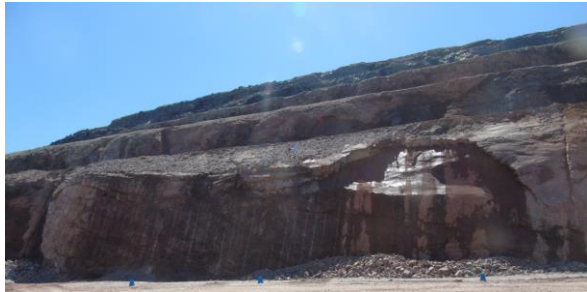
Figure 5. Slope failure and slabs observed on the southeast wall (bench 700-728)
