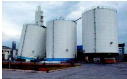
Figure 2. Overturning failure of a circular storage tank due to the lack of bearing capacity (API 2001)
