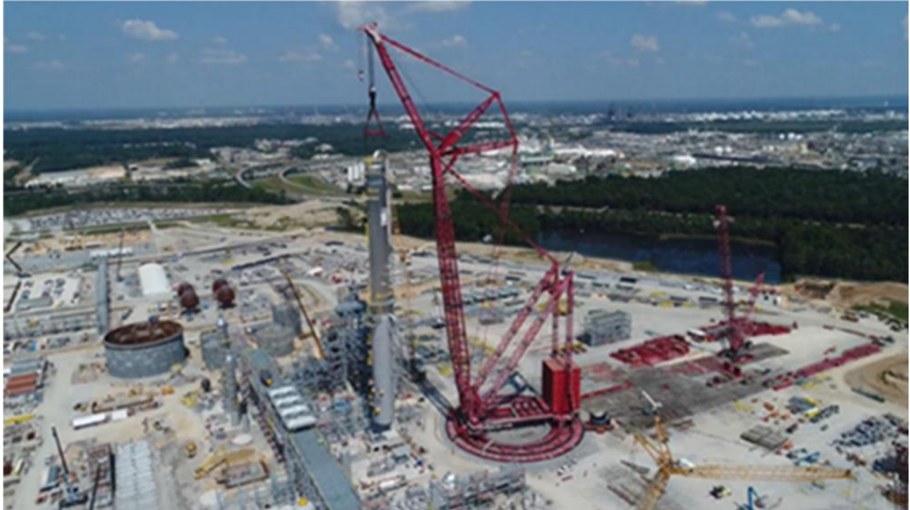
Figure 13. On site photo of wash tower lift with PTC-200 DS ringer crane (courtesy of Mammoet Fabrication B.V.)
