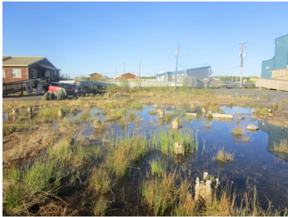
Figure 1. Timber piles that were severely decayed such that the houses had to be demolished. Photo taken in Inuvik, NWT.
