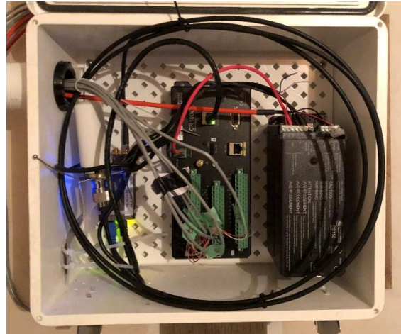
Figure 8. Cellular modem, data-logger, and battery (left to right)
