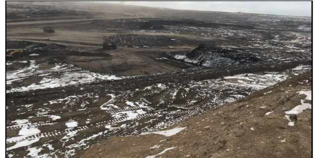
Figure 9. Photo taken from ore crest showing the open cut and buttress construction.
