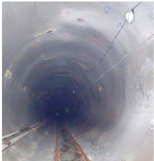
Photo 10. Downstream portion of the T2 tunnel, excavated by a tunnel boring machine (J. Morgenroth)
