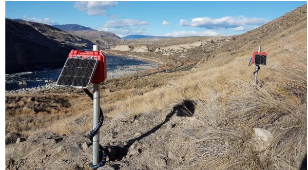
Figure 7. Low-cost datalogger installation at Ripley Slide near Ashcroft, British Columbia
