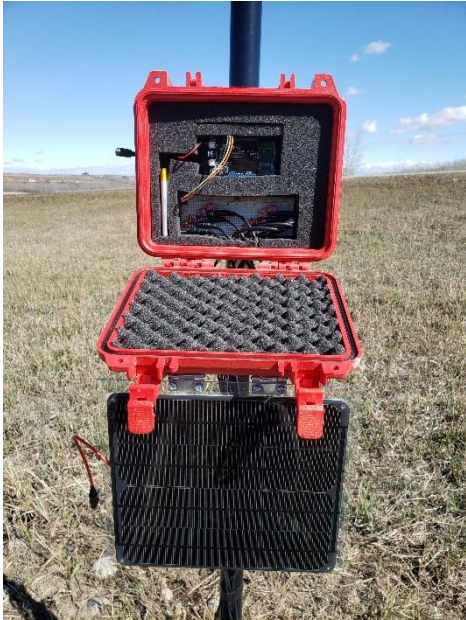
Figure 8. Accessing data from low-cost datalogger installation at Borden Bridge
